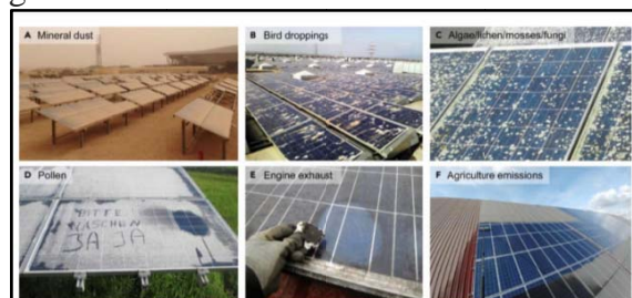
Figure 4 : Possible soil and dust- deposition on PV module
